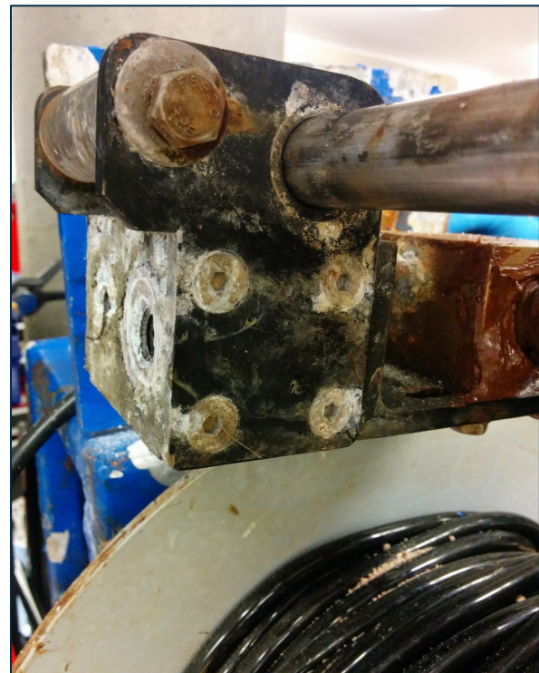
Vital buoy winch parts wear out due to being in a seawater environment 24x7x365.
